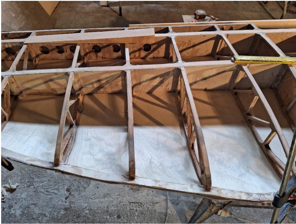
Above: Leading Edge ribs in place and bottom skin, but no LE ply yet.
